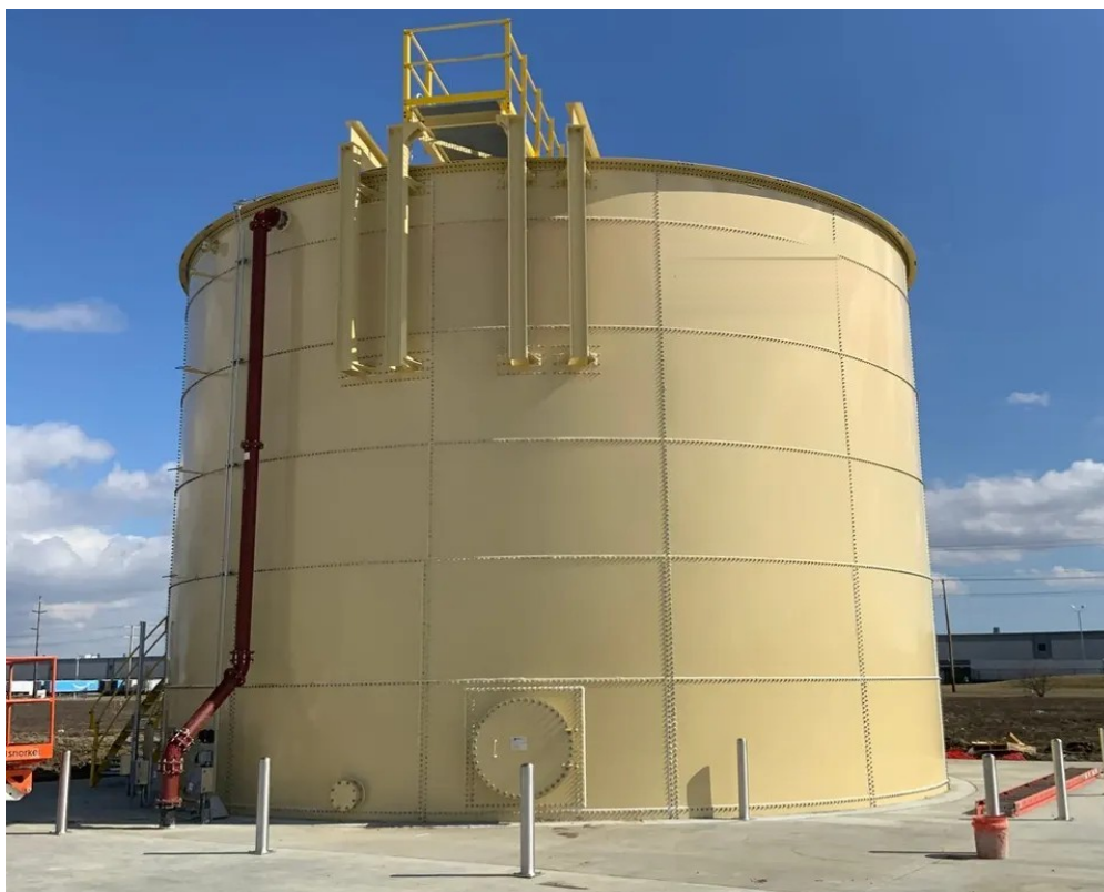
Factory-coated bolted steel tank in industrial service — roof access platform, exterior riser, shell manway and bollard-protected apron
